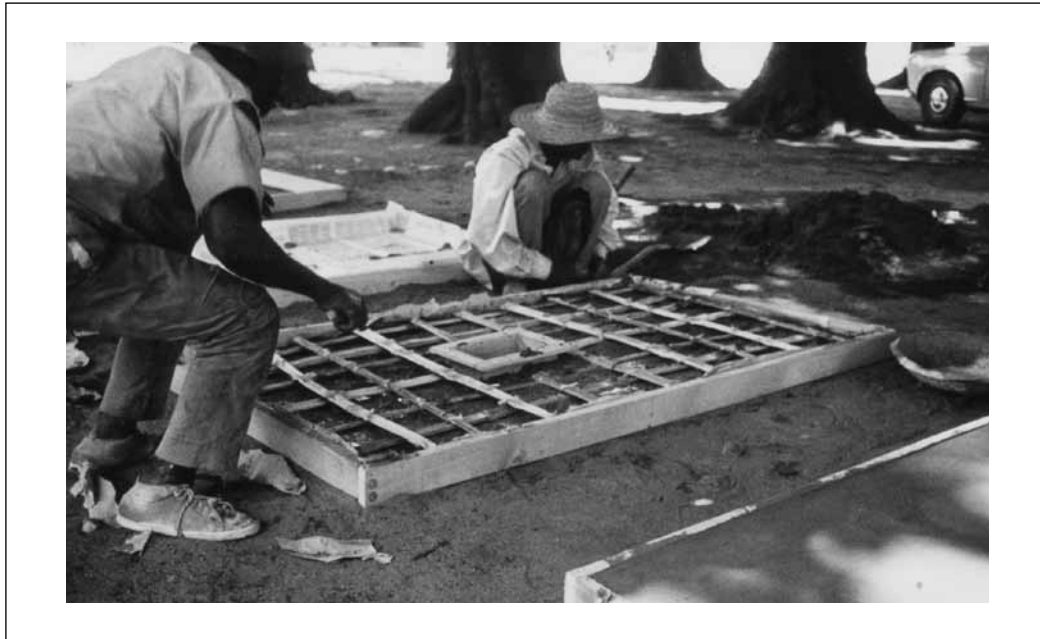
Latrine construction, Ifakara, 1974–1976, “method Eichenberger”, source: SWISS TROPICAL AND PUBLIC HEALTH INSTITUTE (SWISS TPH)
